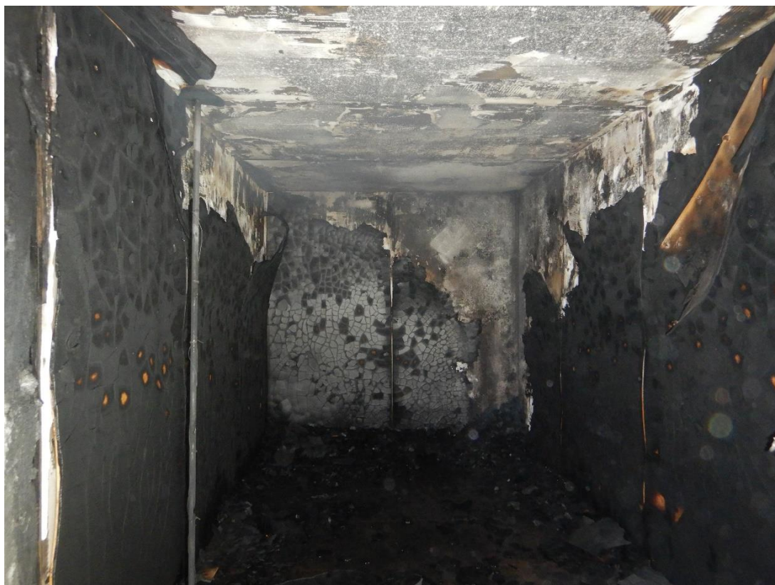
Figure 18 The system at the end of the reaction-to-fire test.
